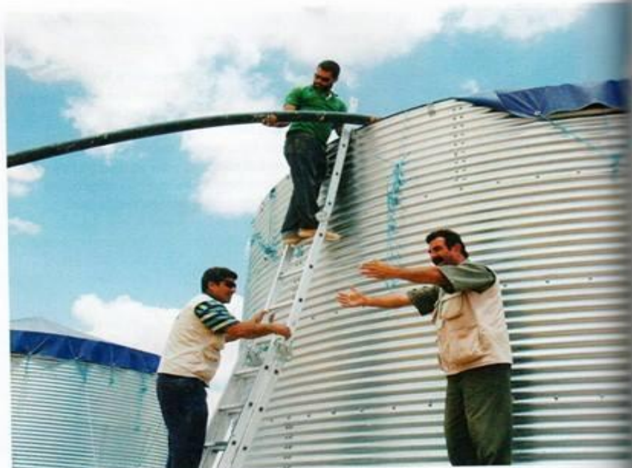
Oxfam public health staff add the finishing touches to 95,000 litre water tanks to increase the water storage capacity in the Za'atari refugee camp in Jordan
