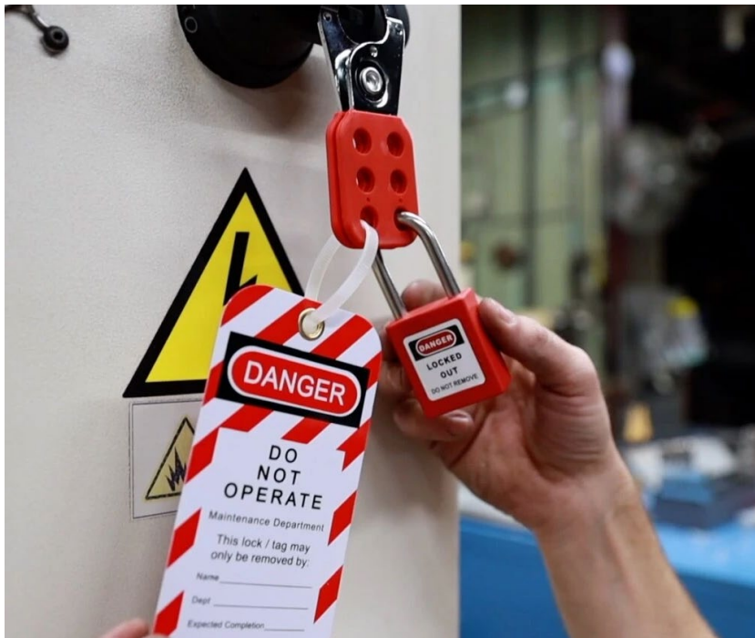
Figure 6-10: Logout – tagout system in place 33
