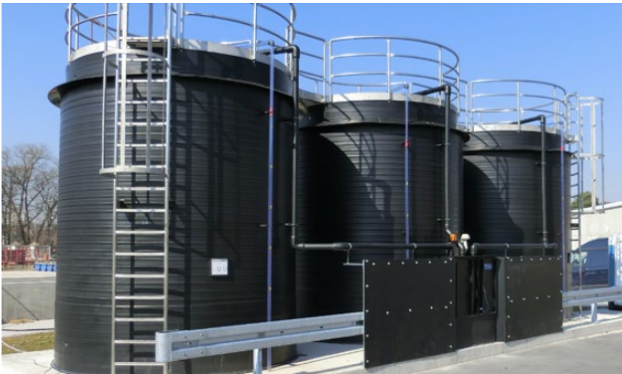
Figure 2-58: Double-walled HDPE tanks 36
